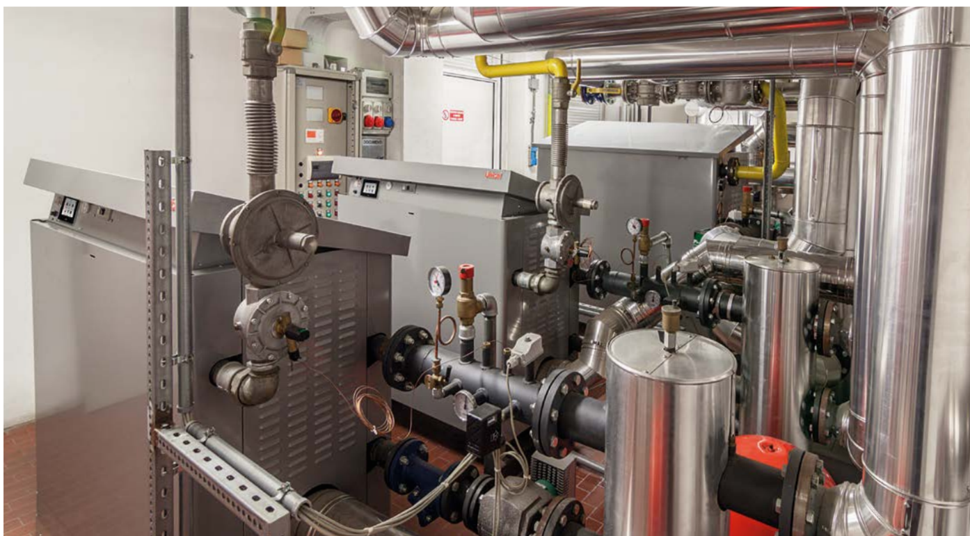
INSTALLATION IN BOILER HOUSE
